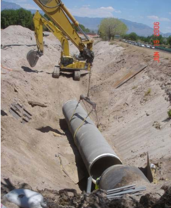
Figure 8. Raw water pipeline (72 inch) - looking east along Paseo del Norte
