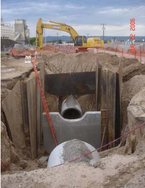
Figure 11. Raw water pipeline #2 72-inch RCP, pipe cradle support for raw water drop manhole
