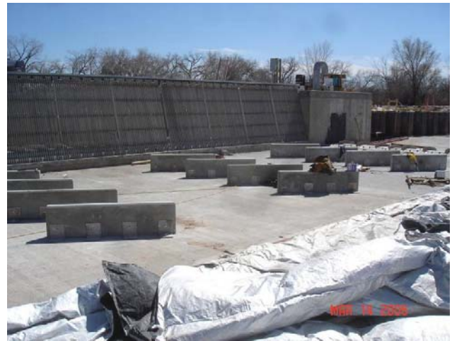
Figure 4. Diversion dam - intake screens and Iowa vanes
