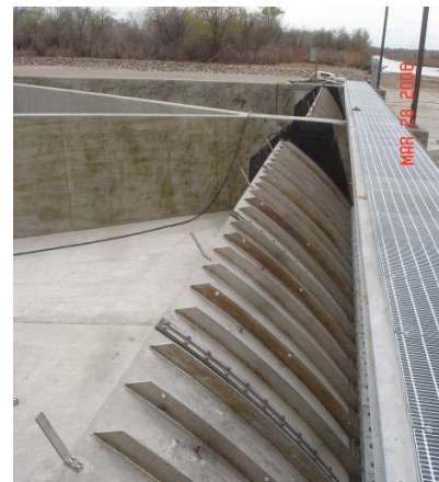
Figure 5. Diversion dam intake control gates
