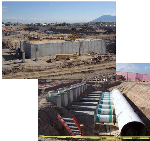
Figure 19. Settled water pump station (left); Rapid mix inlet (right)
