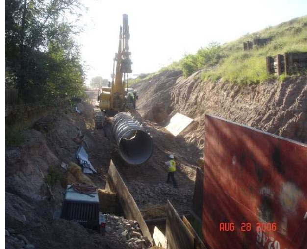
Figure 13. Raw water pipeline #1 delivering carrier pipe to east side of 2nd Street bore
